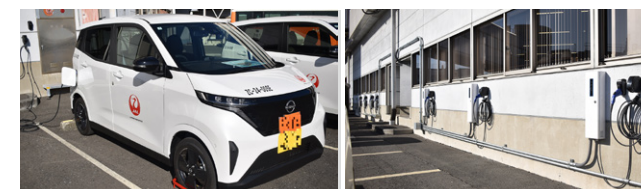
EVs and Charging Infrastructure Provided as an Integrated Solution
