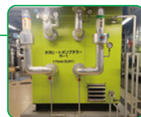
Geothermal heat pump chiller
