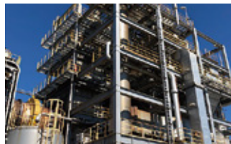
Waste incineration facility
