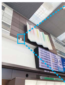
LiDAR installation status
