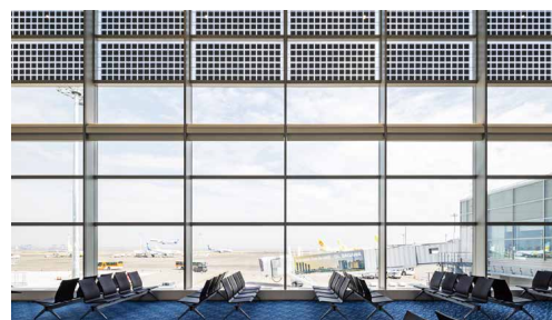
The installation (interior)
